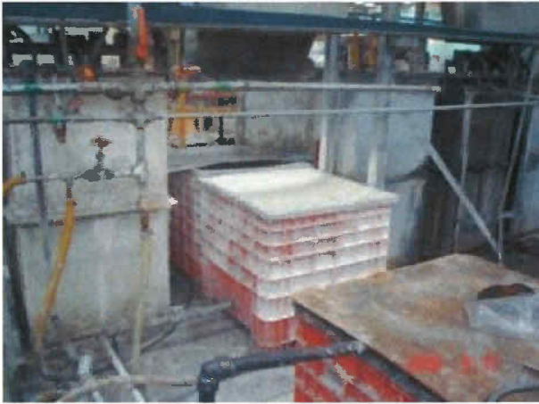
Figure 3: Corroded floor beneath the plating operation . Clarifier sumps were used to contain plating fluids and acids.
