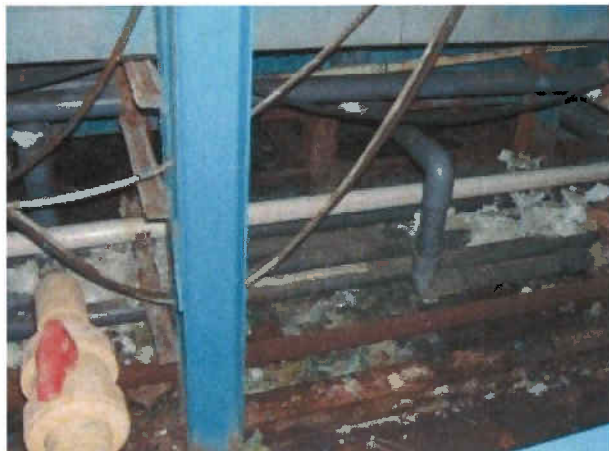
Figure 1: The concrete floor beneath the plating operation was visibly corroded and in poor condition.
