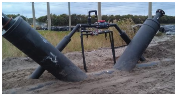
Gas header cleanouts with isolation valves
