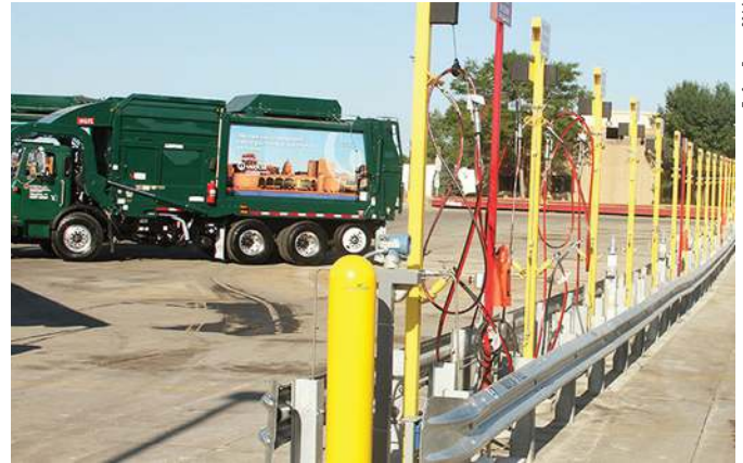
Exhibit 2. Time-Fill CNG Station
