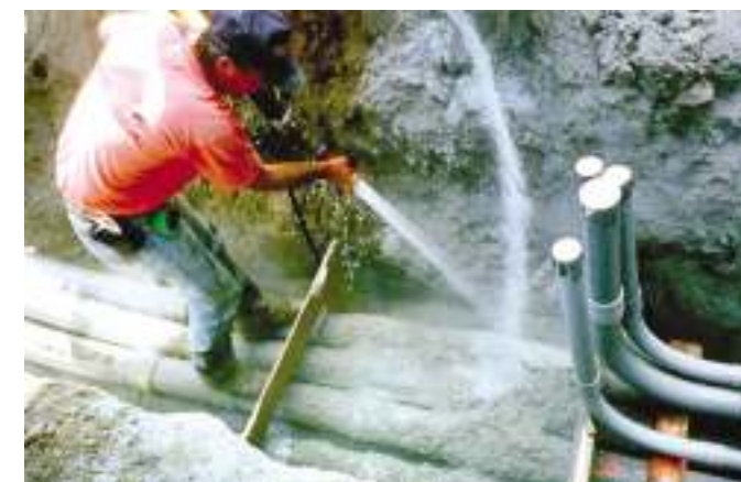
A bentonite slurry dam is being installed in a utility trench to prevent gas migration
