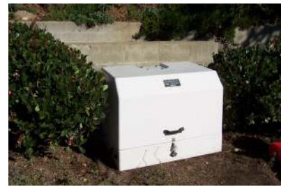
Stormwater monitoring stations can be housed in small, locking weather-proof enclosures.
