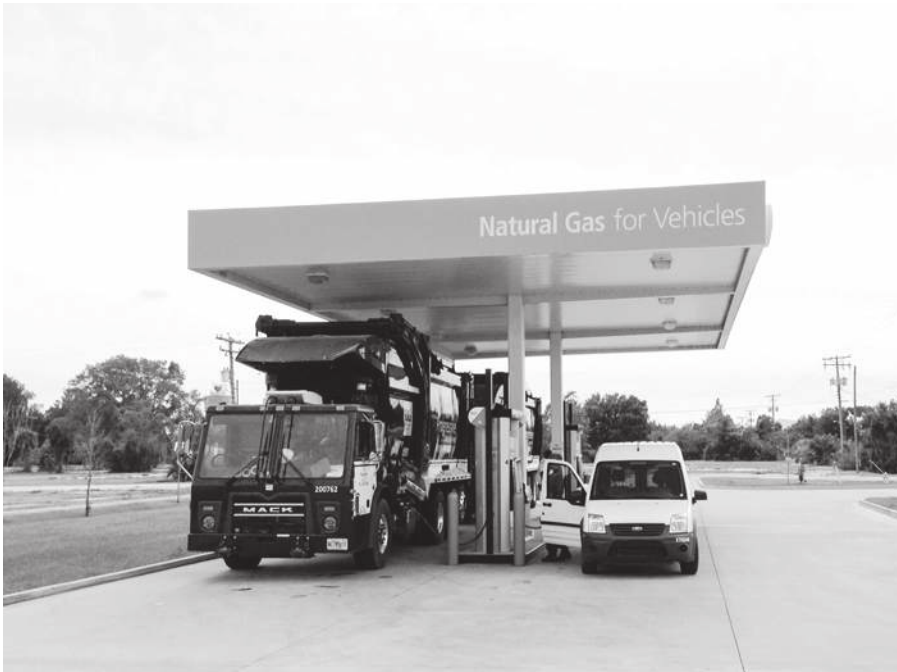
Fast-fill CNG station designed to accommodate two types of vehicles, Tampa, Florida
