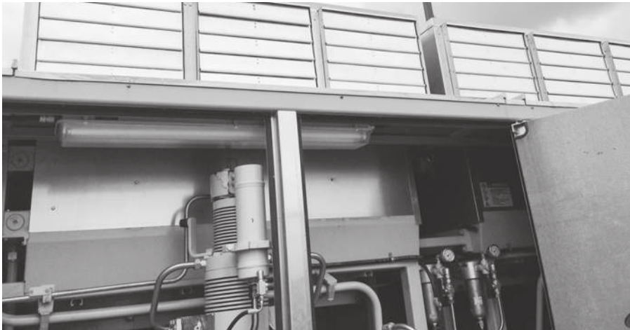
Enclosure designed to buffer compressor noise, Tampa, Florida
