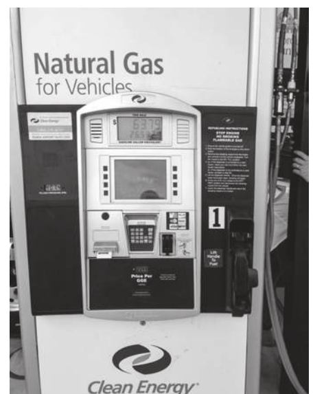
Card reader system, Tampa International Airport CNG Facility, Tampa, Florida
