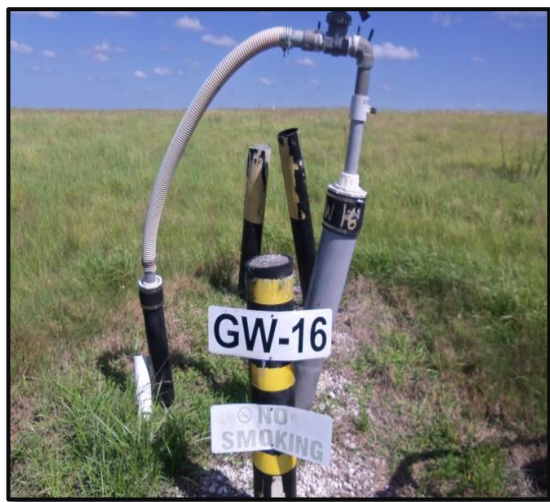
TYPICAL VERTICAL EXTRACTION WELL INCORPORATED IN BEE RIDGE LANDFILL'S GCCS.
