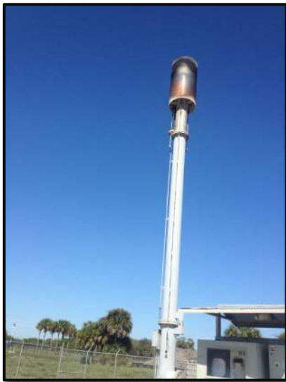
PICTURE OF THE FLARE AT BEE RIDGE, WHICH IS PART OF THE LANDFILL'S GCCS.
