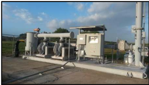
VIEW OF THE FLARE SYSTEM AT BEE RIDGE LANDFILL.
