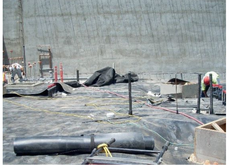
A geomembrane liner system is being installed at the future site of an occupied structure.
