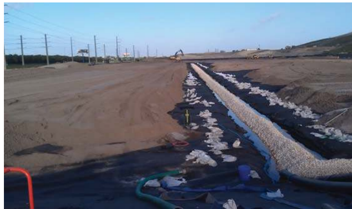
Photo 2: Gravel formed around the pipe Photos courtesy of SCS Engineers
