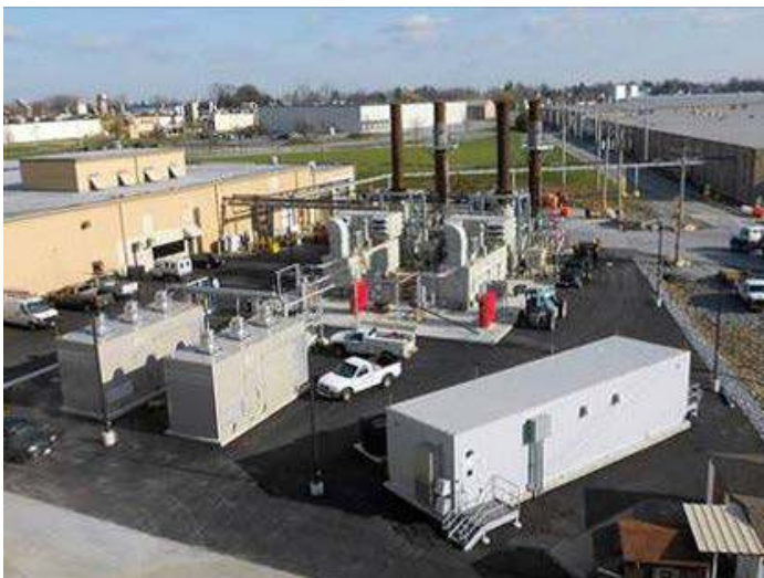
A landfill gas collection system, pictured here, captures methane that can be used to produce electricity.
