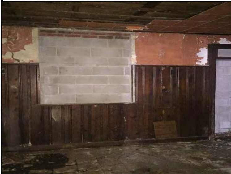
Photo 3: Room 8 - Asbestos Containing Brown Speck 9x9 Floor Tile
