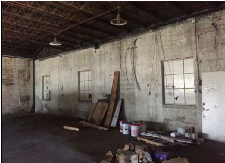
Photo 1: Room 1 - Asbestos Containing Window Pane Caulk
