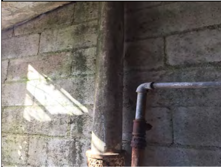
Photo 5: Room 12 - Asbestos Containing Pipe Cement
