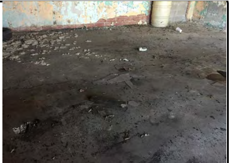
Photo 2: Room 5 - Asbestos Containing Brown 9x9 Floor Tile
