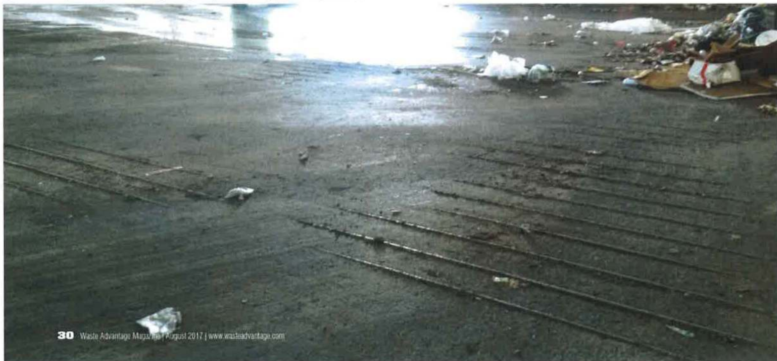
Figure 1: Exposed reinforcing bars signal repair is necessary. Photo courtesy of SCS Engineers.
