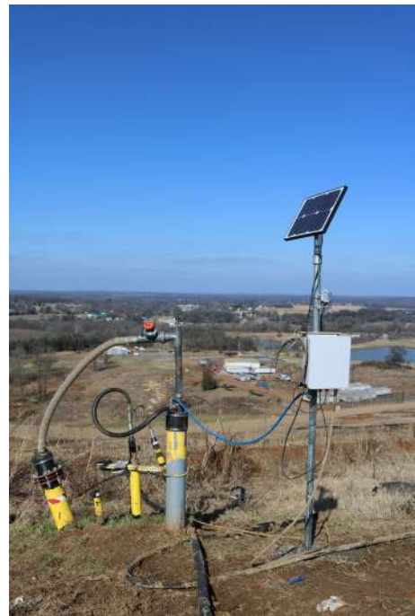
Figure 1 - SCS eTools landfill gas monitoring equipment.
