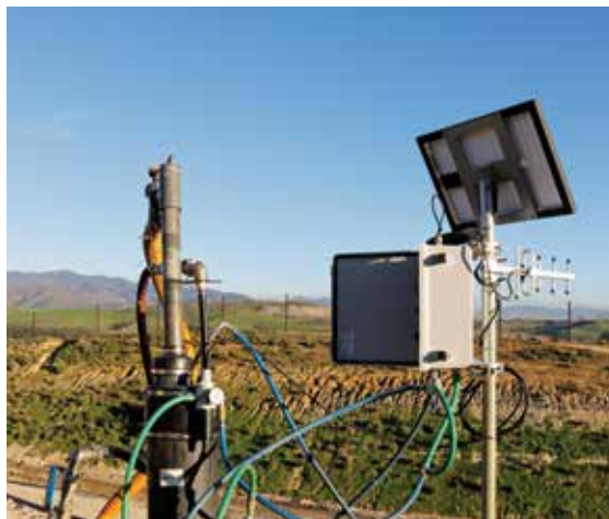
RMC systems allow users to better monitor and control their sites through more interactive features.
