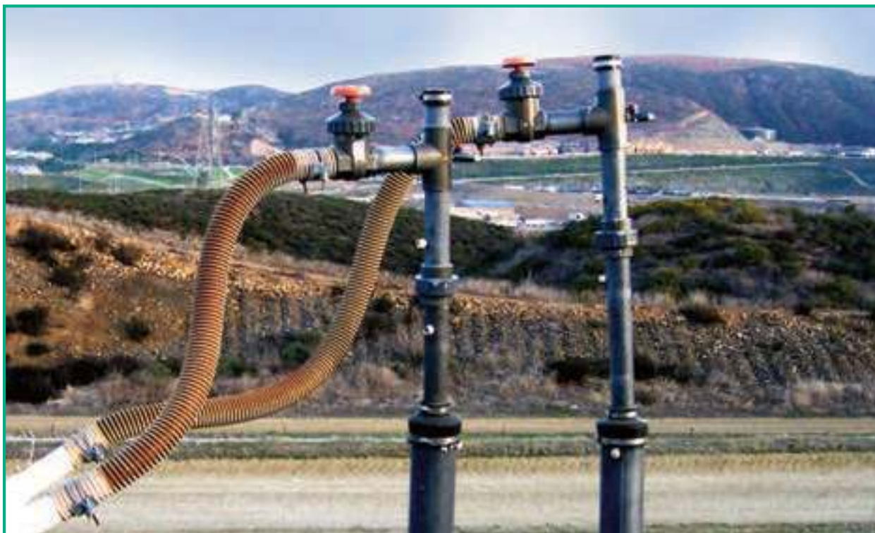
Figure 1. Landfill gas extraction wellheads.
