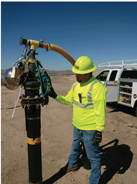
Credit: SCS Engineers Onsite monitoring of LFG equipment
