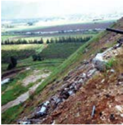
Figure 1: Steeply sloped landfill—difficult to maintain and poses safety challenges
