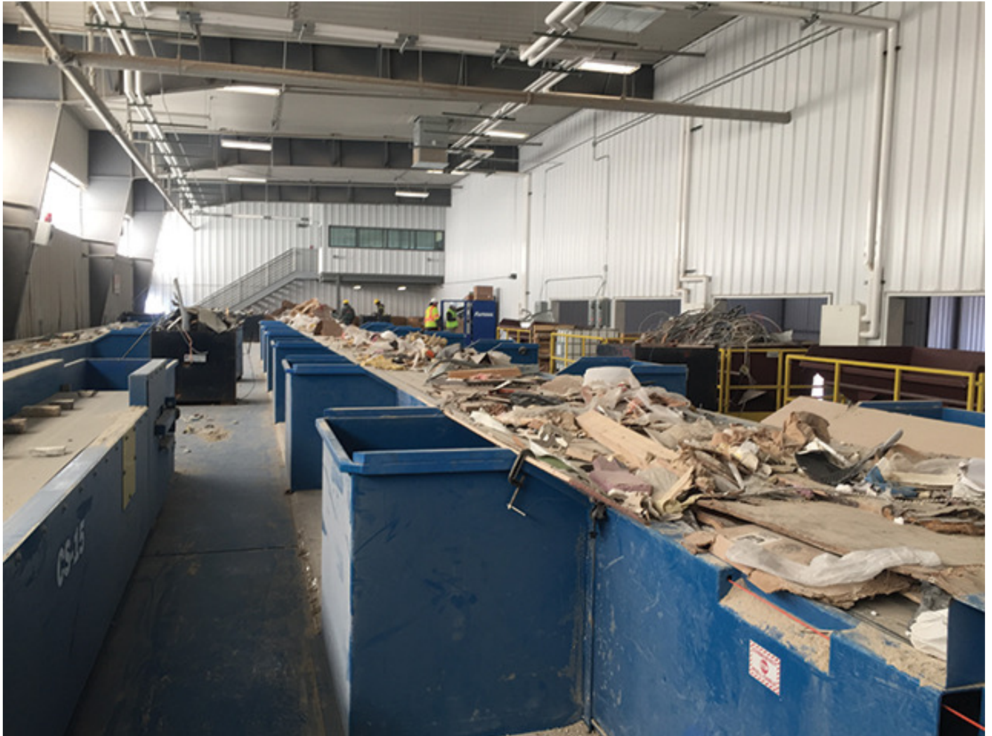
A picking station with access to an emergency pull cord
