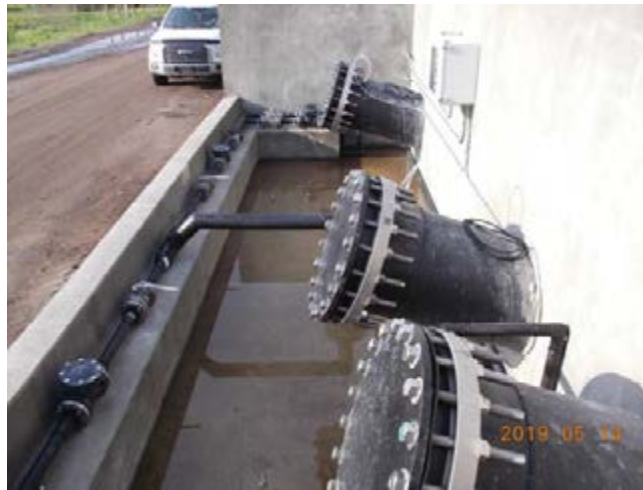
Figure 1 - Leachate removal station with risers and submersible pumps inside risers.
