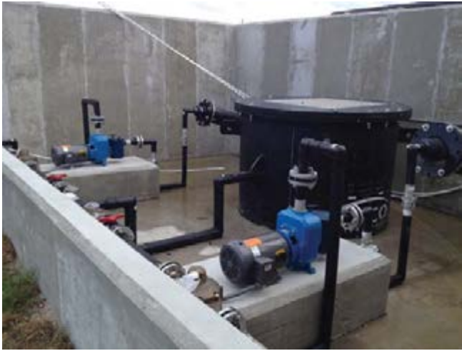
Figure 2 - Leachate removal station with self-priming pumps at the top of the perimeter berm.
