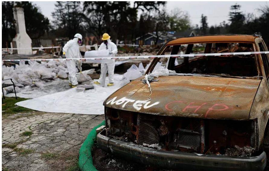
U.S. Army Corps of Engineers contractors in protective gear remove hazardous materials from a home which was destroyed in the Eaton Fire, near a burned car marked “Not EV,” on March 26, 2025 in Altadena.
