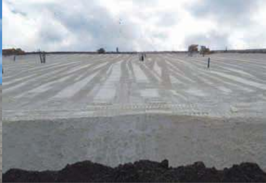
Preparation of slope prior to installation of final cover geomembrane. All gas pipes, well casings and condensate sumps are too short and extensions are required.
