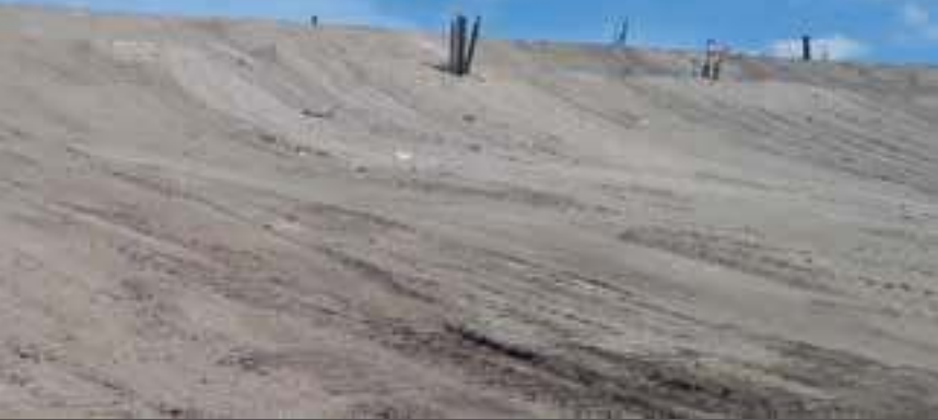
Gas well located near the top of the berm for a tack-on swale, a location conflict.
