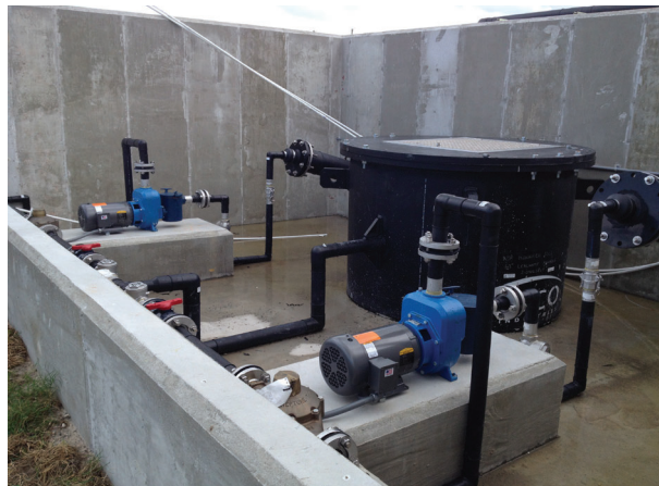
Constructed leak detection system using a dry manhole.
