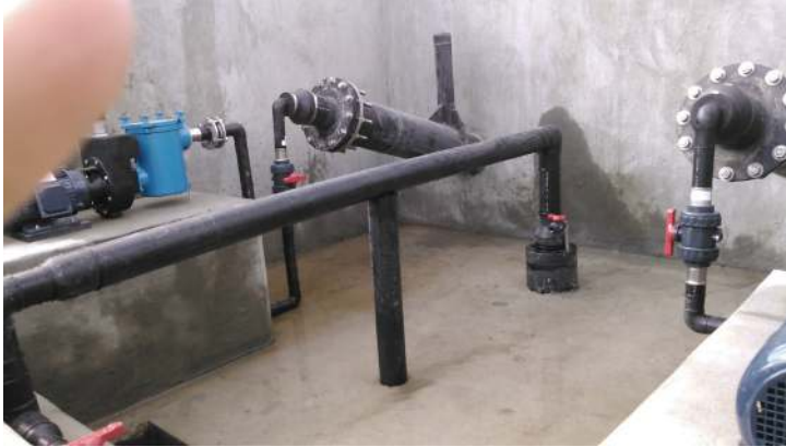
Constructed leak detection system using a valve on casing pipe.
