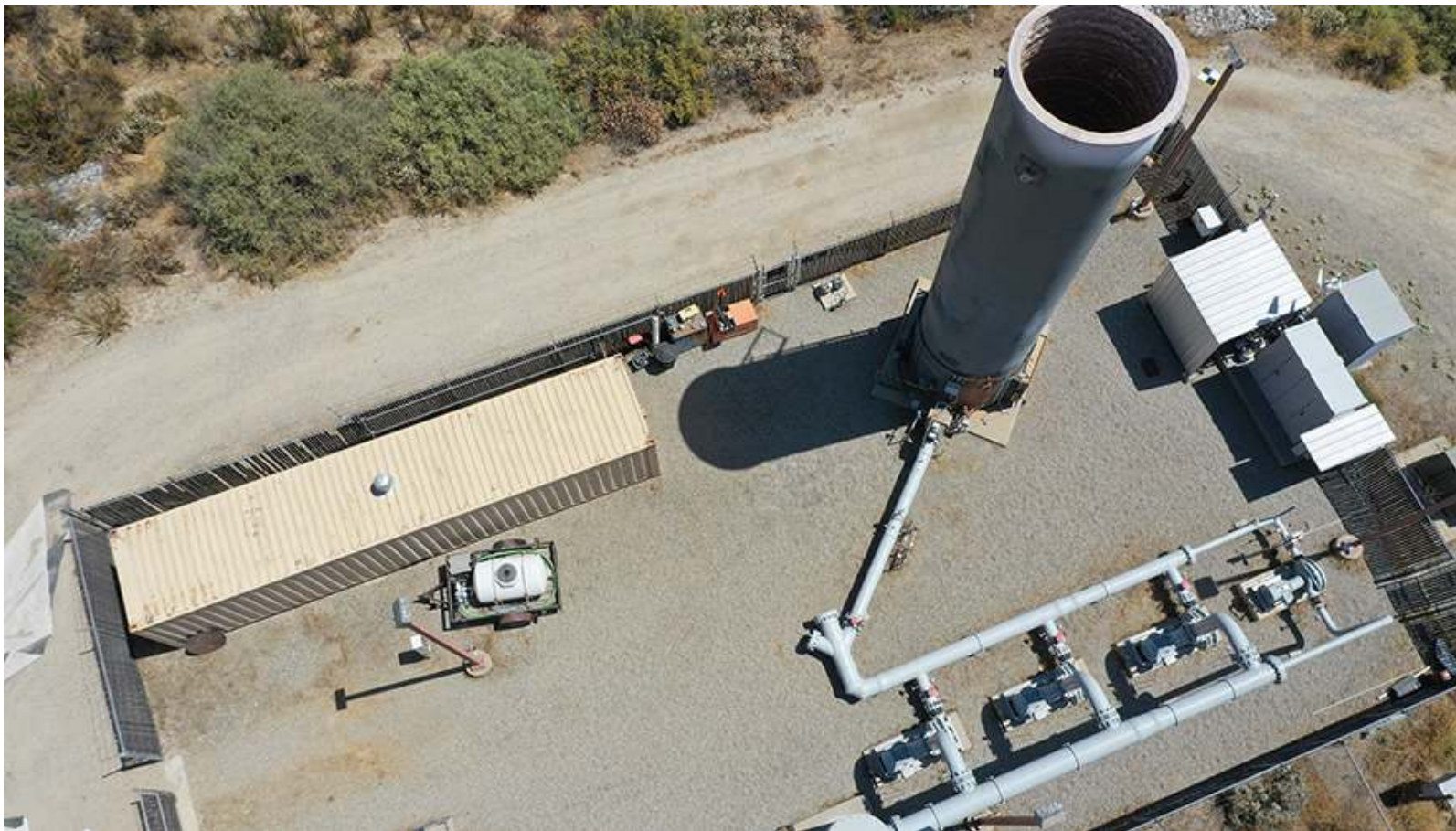
Figure 1: San Bernardino County's almost 500-acre San Timoteo landfill recently upgraded to gas monitoring and controls that manage its four blowers, flare station, pumps, valves, thermocouples and other devices with a pilot project from SCS Engineers, which consisted of 340 tags, 16 screens and more than 50 alarms monitored and managed by Ignition 8.0 web-based SCADA software, Ignition Perspective Internet software module and an Ignition Edge gateway from Inductive Automation. Source: SCS Engineers and San Bernardino County
