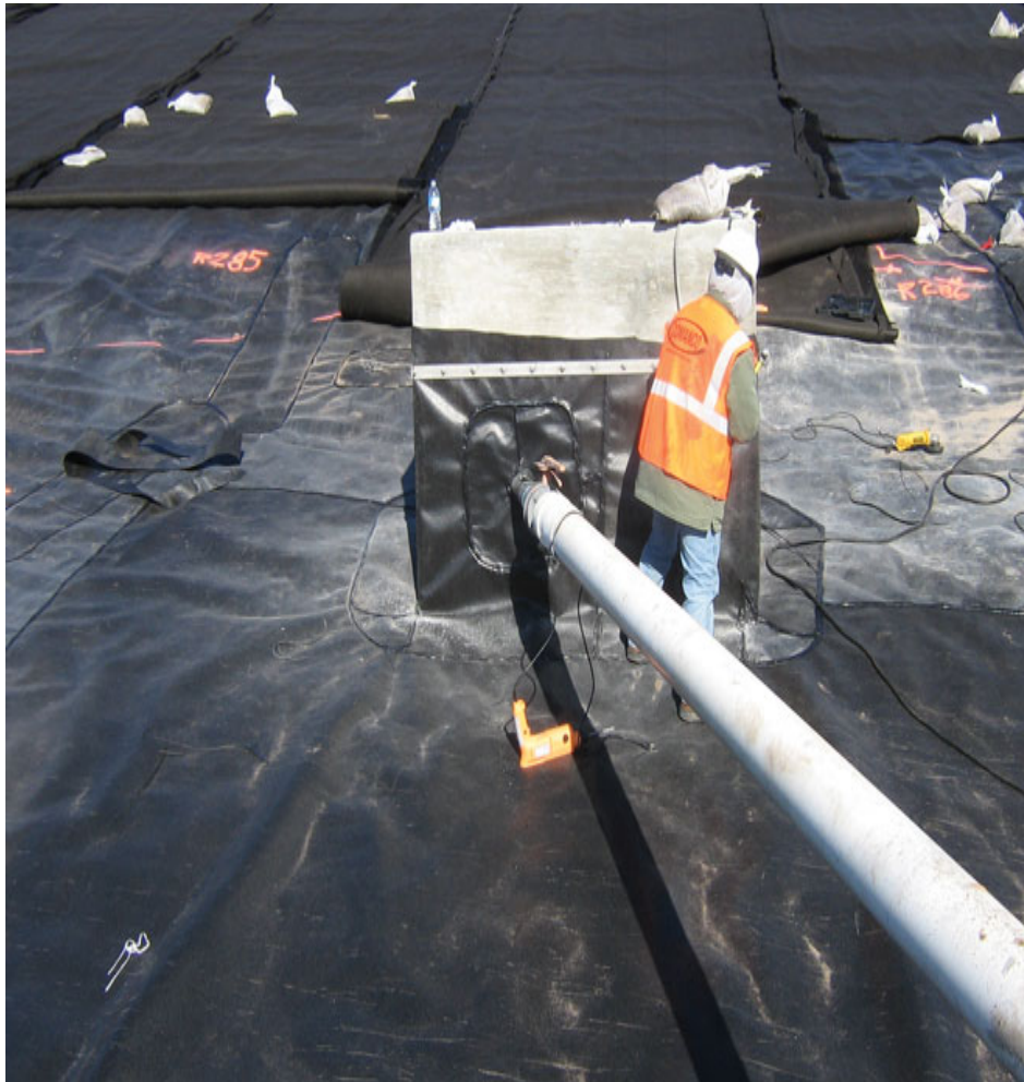
Installation of the final cover geomembrane and attachment to leachate collection manhole.
